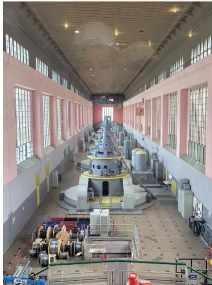
The machine room
